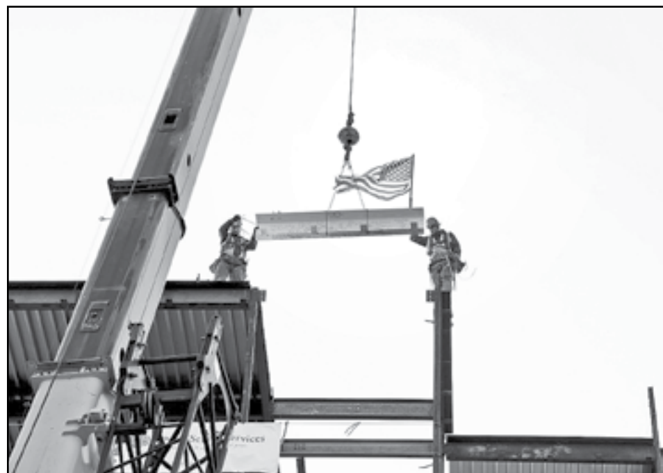
Steel workers placed the last beam onto the new Jewish Senior Services building during the topping-out ceremony on January 22. (Photos by Regina Madwed, Capitol PhotoInteractive)
