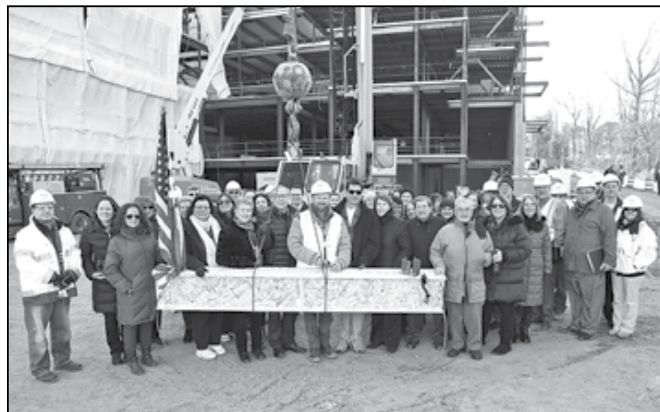
The last steel beam signed by hundreds of Jewish Senior Services board members, volunteers and employees, and KBE Construction employees and contractors just before being raised to the top of the new Jewish Senior Services building scheduled to open in spring 2016.
