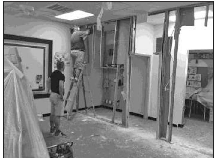
A huge shout out to Frank Floyd and the many volunteers who have been here to help him with our KJDS summer construction projects, which were needed in response to our growing enrollment!
