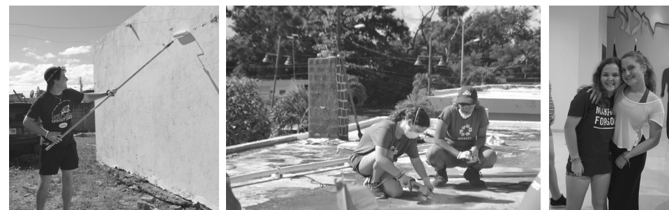
Above: Adam painting, Isabel working on roof repairs, Isabel and Julia during AWB
