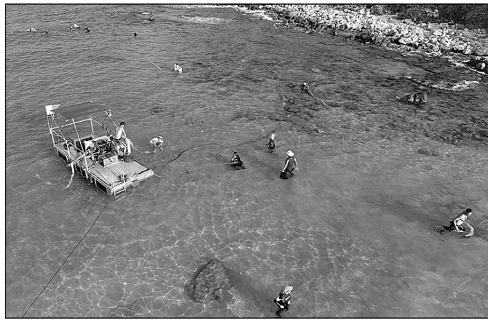
Near shore excavation with a newly developed barge system at the biblical port of Tel Dor, Israel, by researchers at the University of Haifa and the University of California San Diego's Scripps Center for Marine Archaeology. (Photo by Anthony Tamberino/SCMA)
