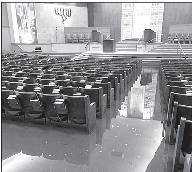
Standing water in Houston's Congregation Beth Yeshurun synagogue following Hurricane Harvey. (Photo courtesy of JNS)
