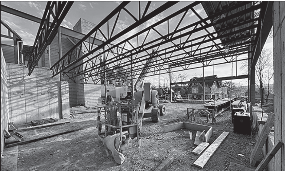
Construction is underway for the Roitman Chabad Center at Cornell University's new building.
