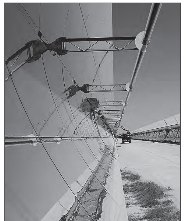
A machine cleaning the parabolic mirrors at the Ashalim Solar Thermal Power Station. (Photo courtesy of the Ashalim Solar Thermal Power Station)
