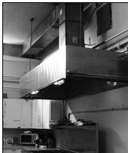
What's Cooking at Temple Israel Manchester? The kitchen renovations are finished! LRC Fire Safety of Manchester installed new duct work to vent the stove and brought our range up to code. Many thanks to Michael Sydney for coordinating the project.
