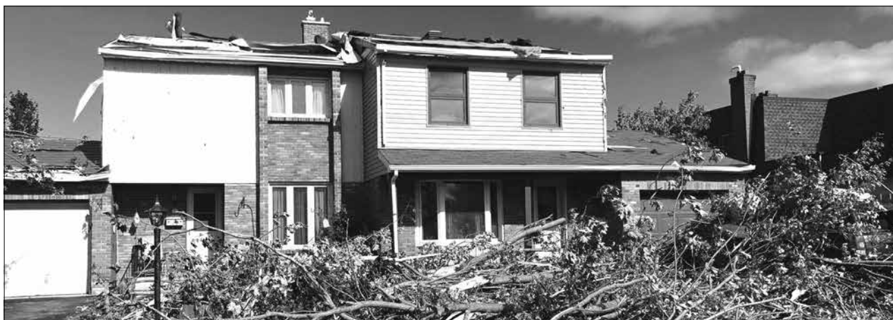
Tornado damage to a home near Greenbank Road is seen in a photo posted to social media.
