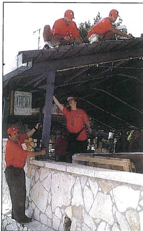
Montreal mission volunteers at work helping to rebuild Café Moment. The café, a trendy coffee shop opposite the Prime Minister's residence in Jerusalem, was attacked by a suicide bomber on March 9, 2002, killing 11 people.
